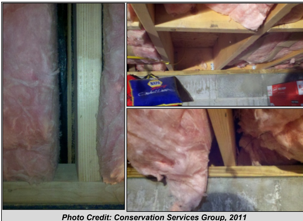
Figure 4- 4: Examples of Grade III (poor quality) Insulation
