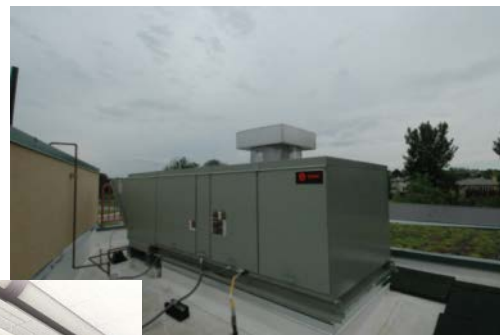
High Efficiency HVAC
