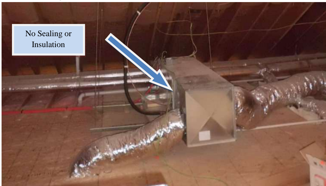
Figure D-21: Uninsulated, Unsealed Ductwork in Vented Attic
