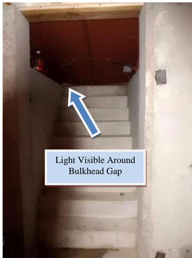
Figure D-19: Basement Missing Door to Bulkhead Hatch
