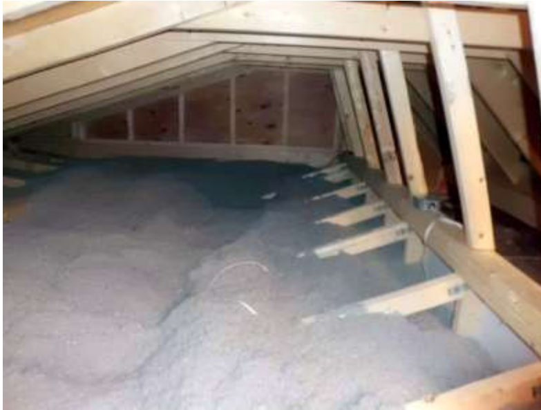
Figure D-13: Uneven Attic Cellulose Installation
