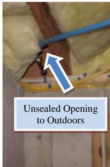
Figure D-7: Uninsulated Rim Joist with Penetrations to Outside
