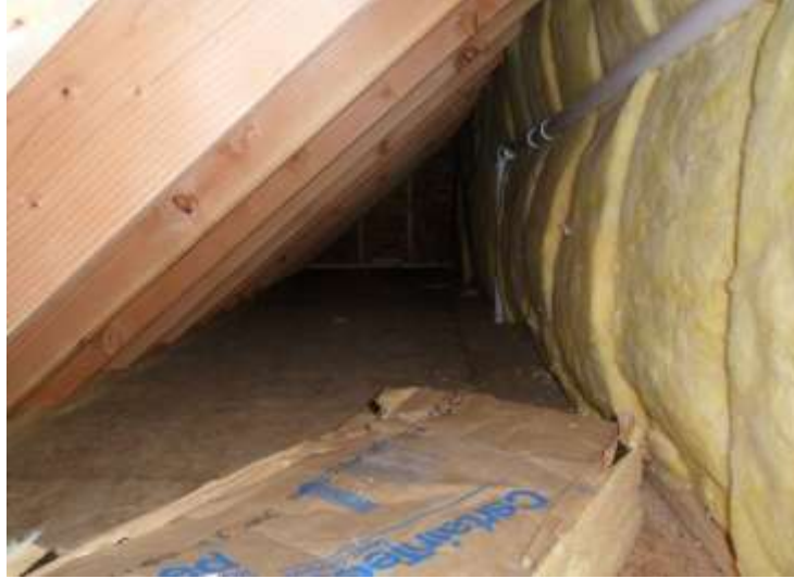
Figure D-16: Knee Wall Insulation Exposed to Wind Washing
