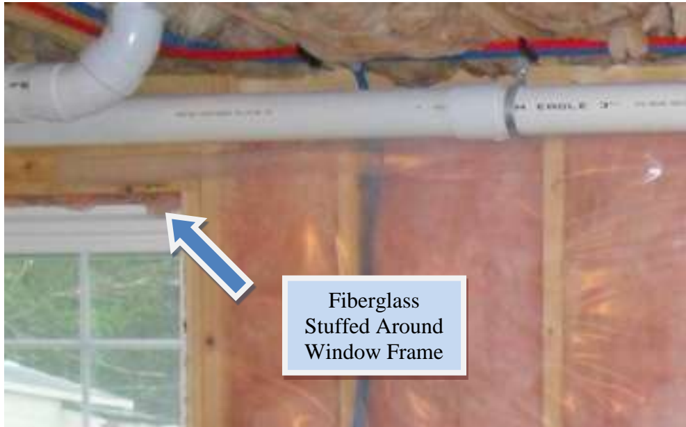
Figure D-20: Fiberglass as Ineffective Air Sealing
