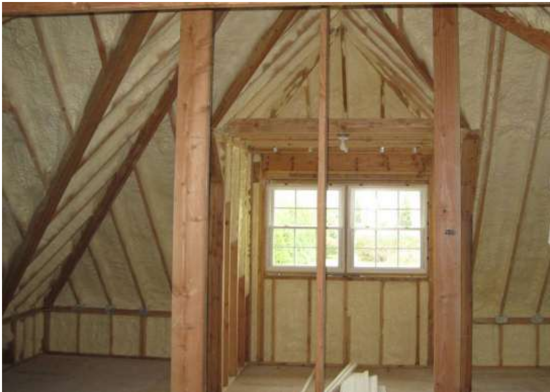
Figure D-9: Walls and Roof Rafters Insulated with Spray Foam
