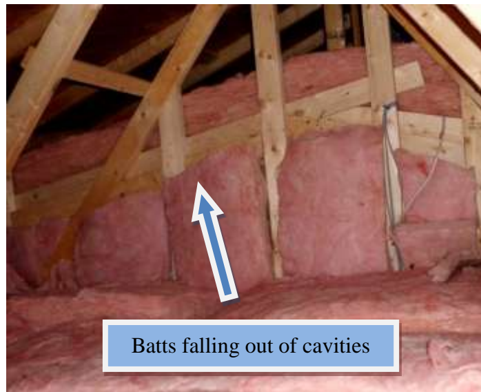
Figure D-17: Poorly Installed Fiberglass Attic Wall Insulation
