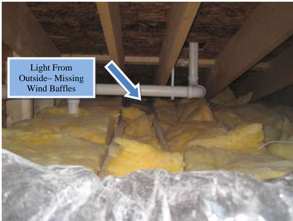
Figure D-12: Poorly Installed Fiberglass Batt Attic Insulation with Missing Wind Baffles
