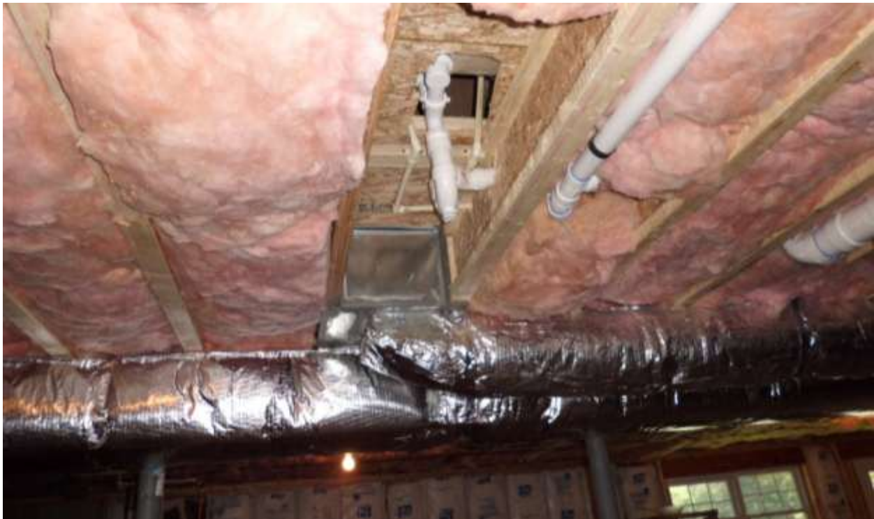
Figure D-6: Missing Frame Floor Insulation & Holes in Subfloor
