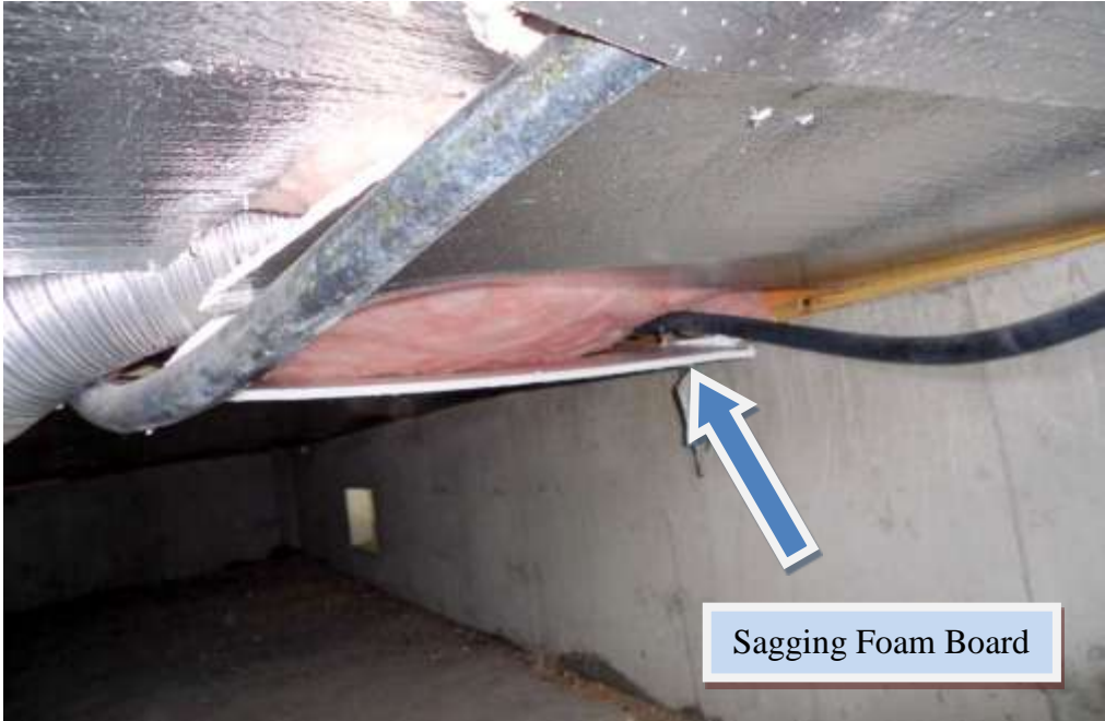
Figure D-4: Crawl Space Frame Floor with Sagging Foam Board Insulation
