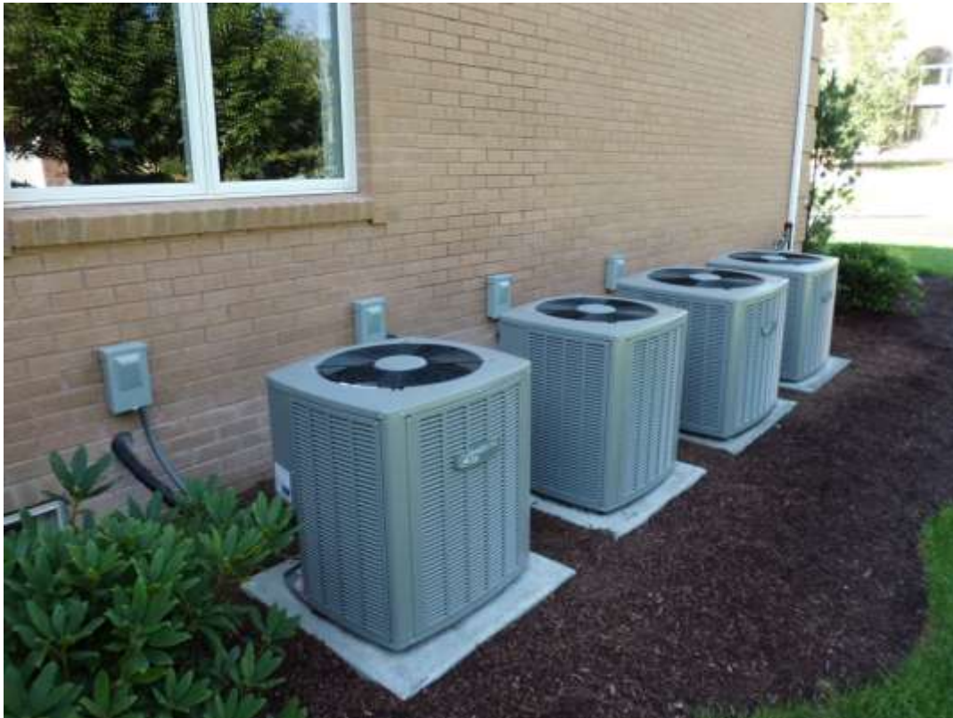
Figure D-24: Large Home with Many HVAC Systems
