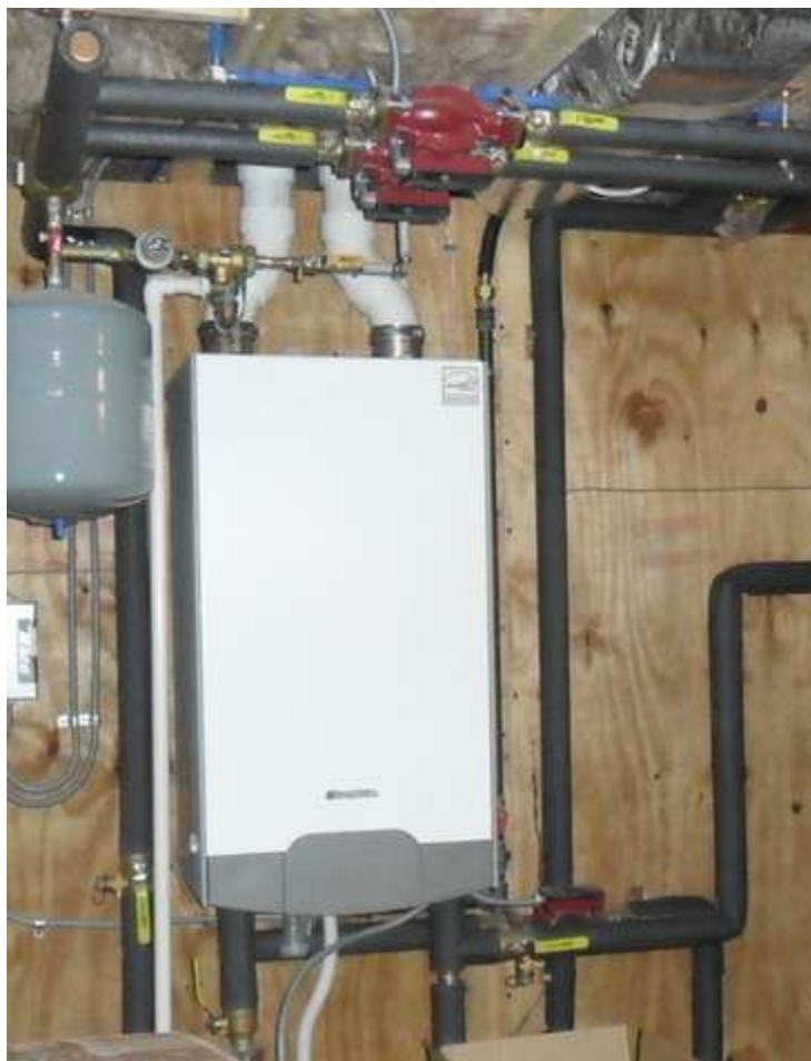
Figure D-25: Well-Installed Hot Water Pipe Insulation
