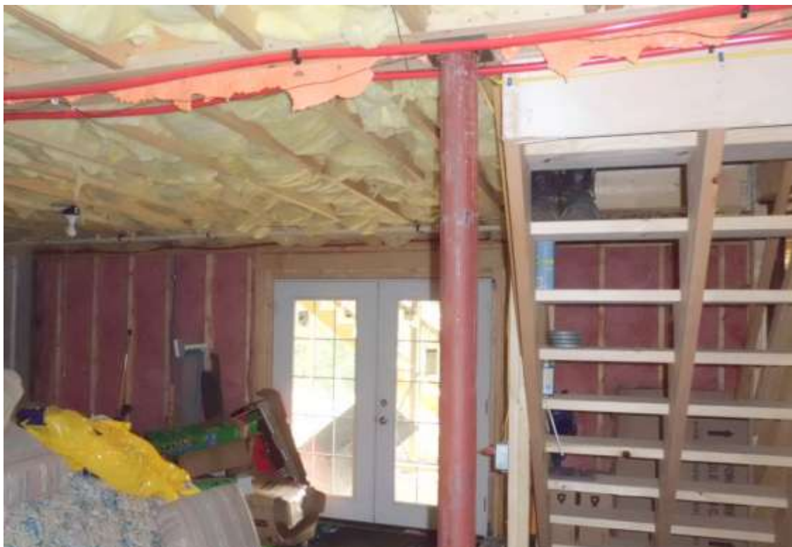
Figure D-5: Poorly Installed Frame Floor Insulation
