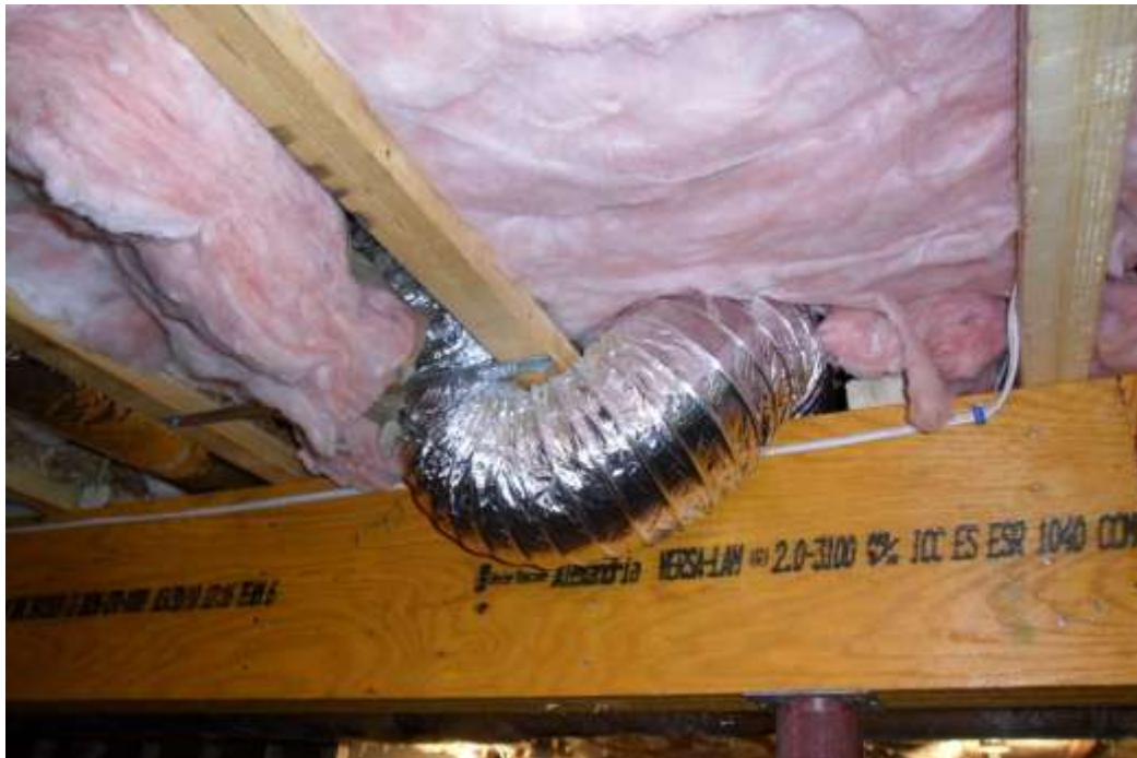
Figure D-23: Kinked HVAC Ducts in Basement
