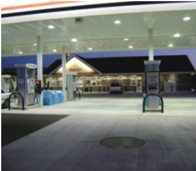
Pre-2009 Canopy Lighting – Metal Halide
